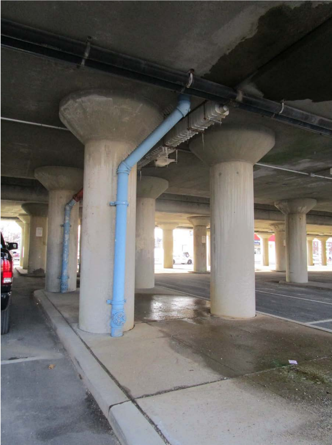
27. LIRR Commuter Parking Lot Water leaking from above, icicles
