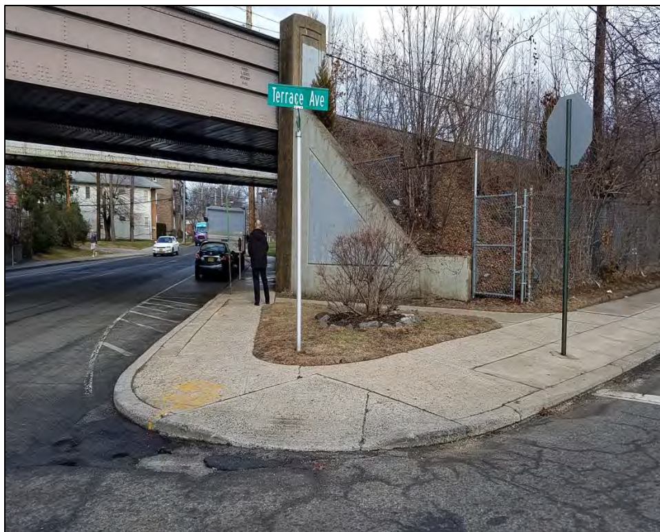
Photo No.: 8 Location: N/E/C Plainfield Ave and Terrace Ave Direction: North Comments: Non-Compliant Ramp; Missing detectable warning strip.
