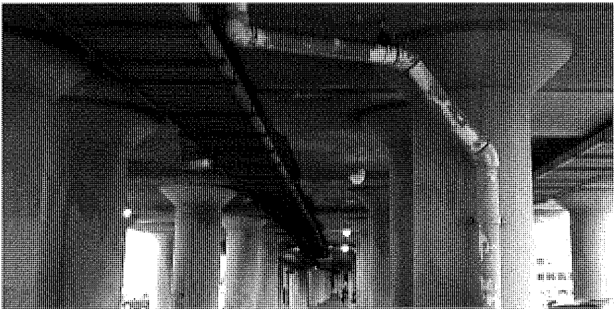
Ineffective pigeon deterrent measures.
