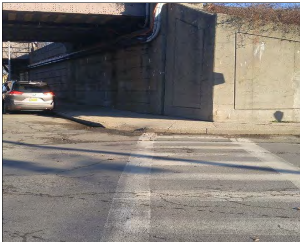
Photo No.: 7 Location: N/E/C Tyson Ave Extension and Atlantic Ave Direction: Northeast Comments: Non-Compliant Ramp; Missing detectable warning strip; Missing ramp.
