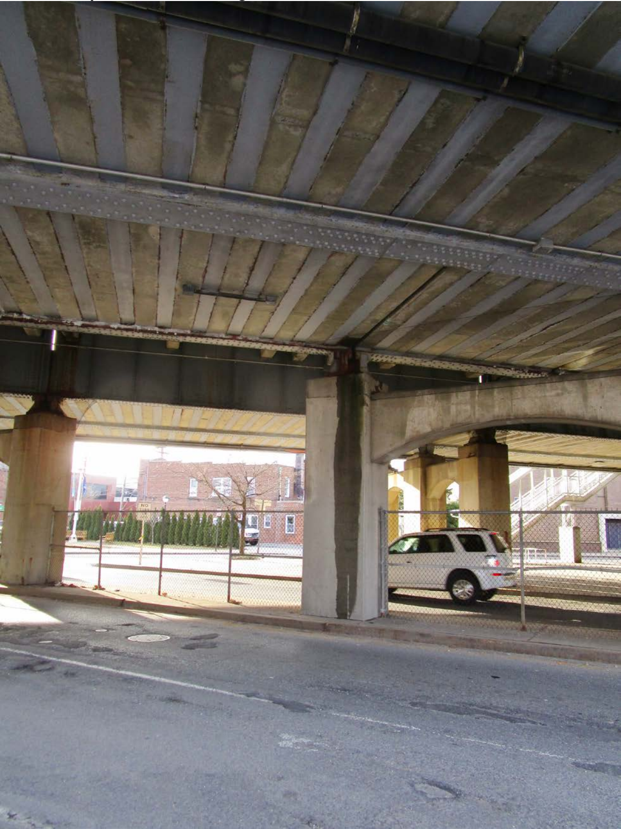
10A. & 10B. LIRR Commuter Parking Lot Pillar at Tulip Ave.; water leaking from above
