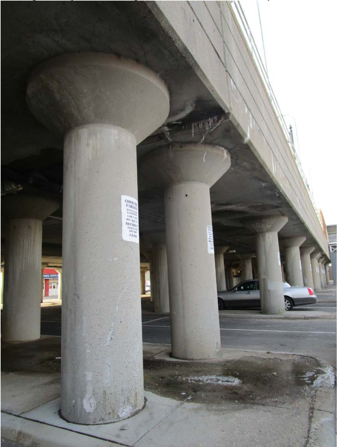
30A & 30B LIRR Commuter Parking Lot Leaking water, puddles—along Caroline Place, west of Tulip Ave.
