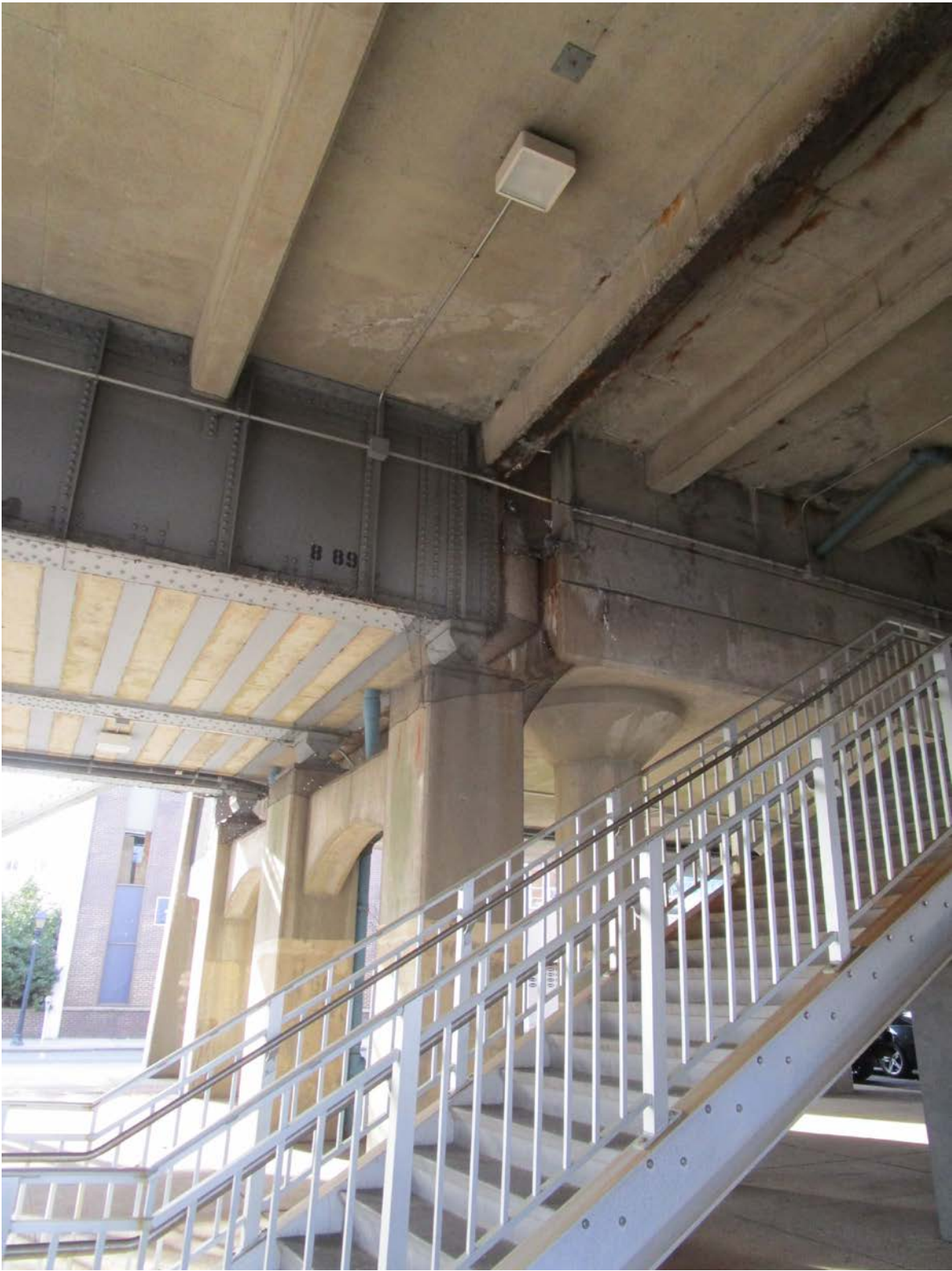
13A. & 13B. LIRR Commuter Parking Lot Staircase - Poor Conditions
