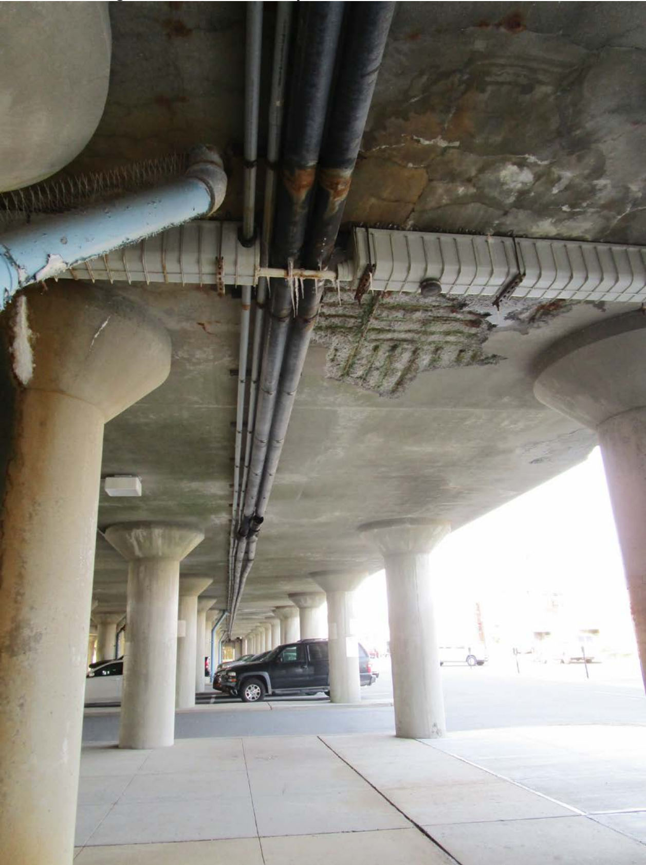
14. LIRR Commuter Parking Lot Rust, crumbling cement above where pedestrians walk
